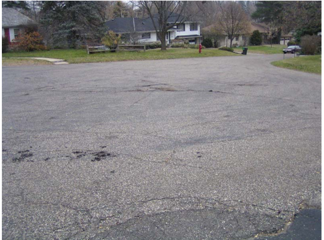
Photo 2. Cracking and Patches
