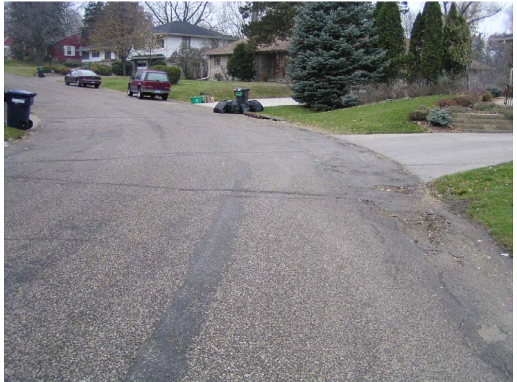
Photo 1. Existing Pavement Condition
