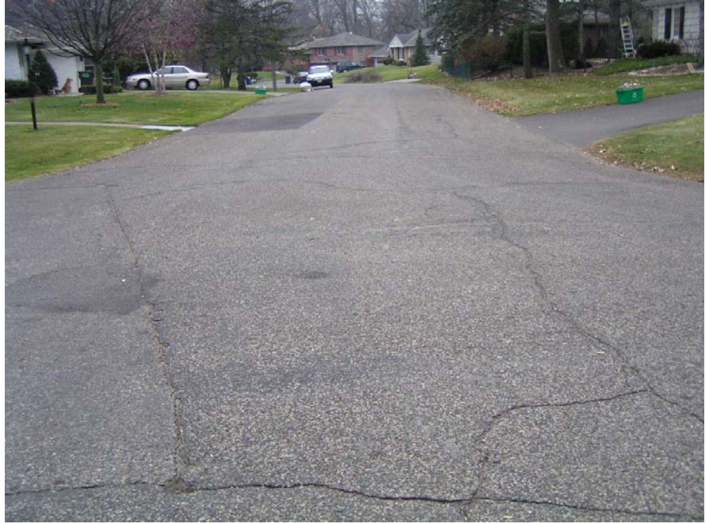
Photo 2. Block Cracking and Patches
